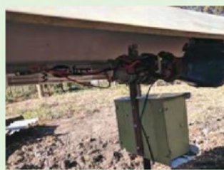
Care Free conditioner installed
