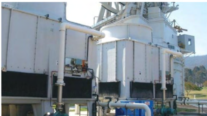
Cooling tower at Canberra Deep Space Communication Complex
