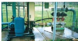
Care Free Conditioner installed into a 150mm line at the golf course. Flowrate: 2700 lit/min Headloss: 41kPa - no orifice.
