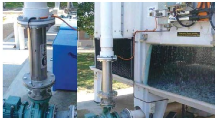
Care Free Units installed directly after pump
