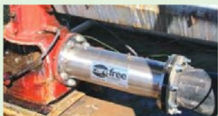
Care Free Conditioner installed at the golf course.
